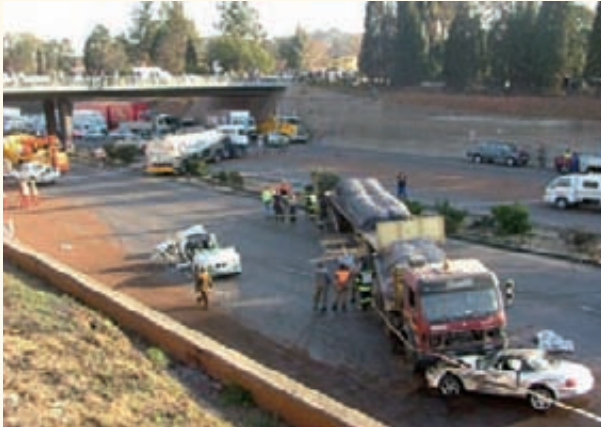
Truck accident on N3 causes considerable road damage, is unsafe for the public, and causes huge delays that influence freight logistics of the country.
