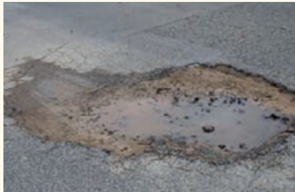
Before blacktop patching
