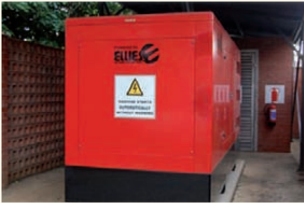
eNaTIS Backup Generator
